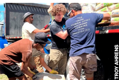
Students and Dennis Borland (right) unload bags of concrete for the construction site at Billy White Primary School.
