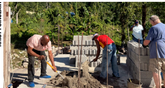
Participants work as a team to lay the foundation for a house.
