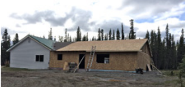
Construction on the new addition to the Tok Church began in May 2018.
