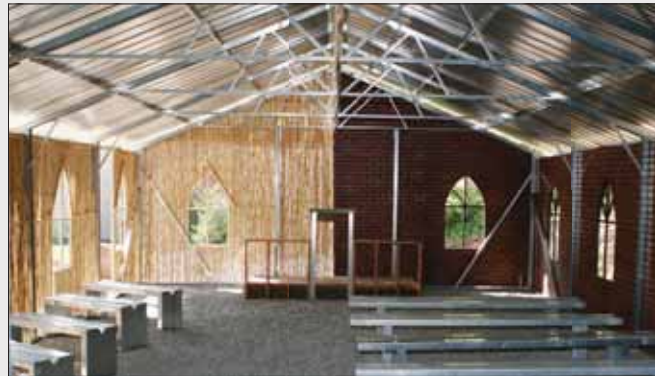
Maranatha and Adventist-Laymen’s Services and Industries are partnering to purchase, ship and assemble (yes, in one day) church buildings in developing countries.
